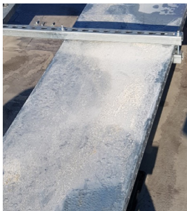
White rust on a cover
